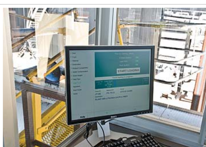
Computer at Load-Out Rack The load-out system incorporates a computer, computer-automated controls, two truck scales, and automated data recording. The automated controls provide remote operation of the asphalt pumps located at the tanks. The load-out controls for each load-out boom incorporates lockouts to prevent operation of the pumps unless the boom is properly positioned and valves are properly set. The components of the truck scales and the load-out system were provided by Astec.
