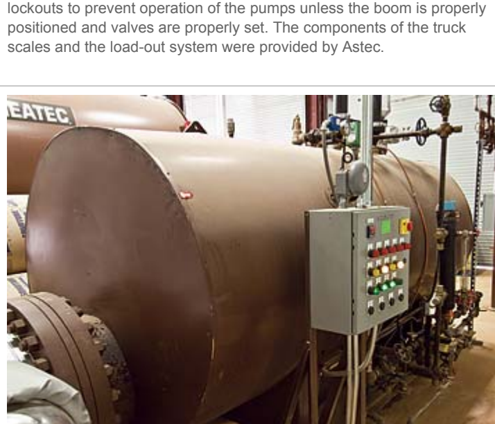
Steam Generator A steam generator turns water into steam—and that steam is used to heat tank cars. The generator is located in the enclosed building alongside the hot-oil heaters. Its source of heat is the thermal fluid that is heated by the hot-oil heaters.
