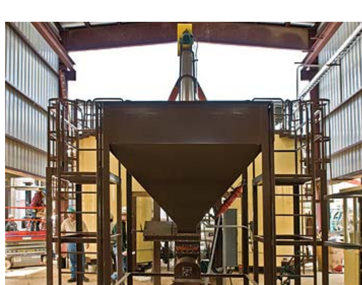
Polymer Blending System The terminal has a separate building that was constructed specifically for housing the equipment needed in the company's polymer blending operations. In the foreground of this photo is the hopper where polymer pellets are loaded. The two tanks in the background are used to mix the polymer with liquid AC. According to a Heatec spokesman, C.W. Matthews Contracting will have processed more than 20,000 tons of polymer mix in the months between May 2009 and the end of the paving season.
