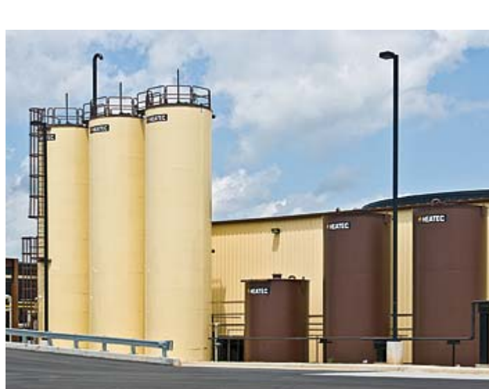
Polymer Let-down Tanks There are three 35,000-gal. tanks that are used to store finished PMA (polymer modified asphalt) at the Rockmart Terminal.
