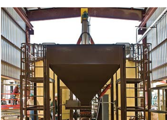
Polymer Blending System The terminal has a separate building that was constructed specifically for housing the equipment needed in the company's polymer blending operations. In the foreground of this photo is the hopper where polymer pellets are loaded. The two tanks in the background are used to mix the polymer with liquid AC. According to a Heatec spokesman, C.W. Matthews Contracting will have processed more than 20,000 tons of polymer mix in the months between May 2009 and the end of the paving season.
