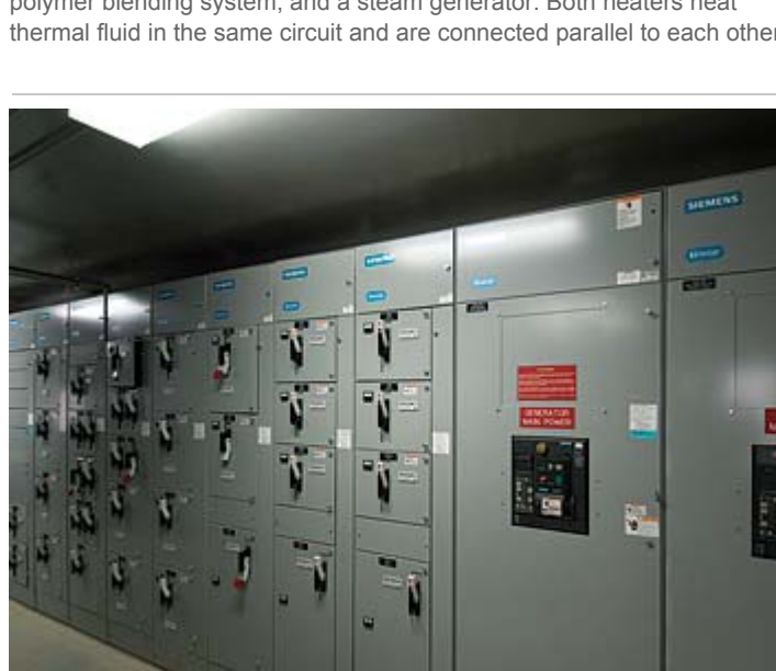
Motor Control Center The control center centralizes all electrical power for the terminal and for the motor controls. The controls are housed in a series of electrical racks and panels. Electrical power is sub-divided into two independent control systems, one for the polymer blending system and another for all other electrical power. A computer is also located in the motor control center. It controls the asphalt pumps used to transfer asphalt from one tank to another. Positions of the three valves on the outlet side of each asphalt pump can be verified on the computer screen before the pump is operated.
