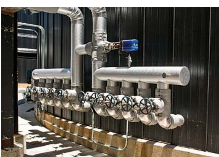
Hot-Oil Piping System The asphalt storage tanks, steam generator, and heat exchanger have independent parallel piping circuits connected to the main supply and return lines. The coils of each tank are separated into independent circuits, each with its own control valve.
