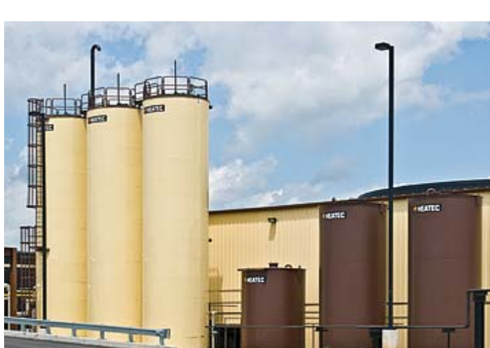
Polymer Let-down Tanks There are three 35,000-gal. tanks that are used to store finished PMA (polymer modified asphalt) at the Rockmart Terminal.
