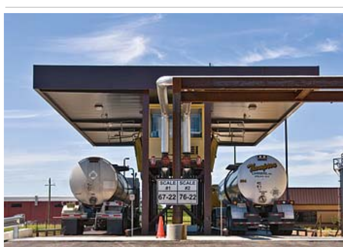
Dual Load-Out Rack The tank truck load-out system is designed so that drivers can safely load the tank truck they are driving without help from others. Two trucks can be filled simultaneously with liquid-asphalt products, each at a rate of 500 gpm. The loading station has a covered roof and an enclosed control room with two sets of operator load-out controls. The system incorporates an overflow device that automatically shuts off the asphalt in case the scales fail to do so when a preset limit is reached.
