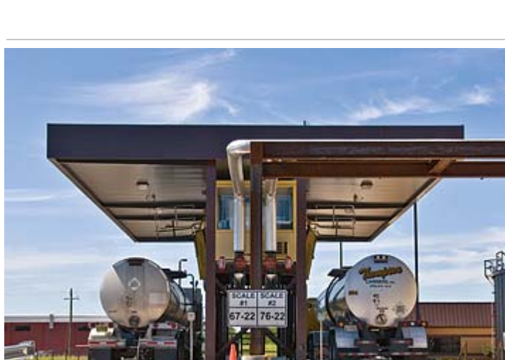
Dual Load-Out Rack The tank truck load-out system is designed so that drivers can safely load the tank truck they are driving without help from others. Two trucks can be filled simultaneously with liquid- asphalt products, each at a rate of 500 gpm. The loading station has a covered roof and an enclosed control room with two sets of operator load-out controls. The system incorporates an overflow device that automatically shuts off the asphalt in case the scales fail to do so when a preset limit is reached.
